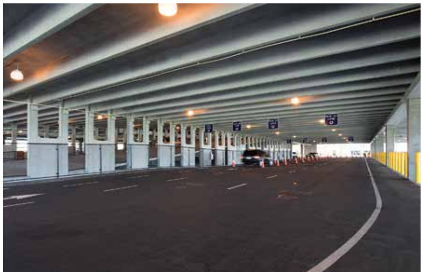
Five 60-foot-wide bays on a 360-foot-long footprint were used for Cruise Terminal One.
